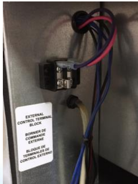
New Terminal Block Location
